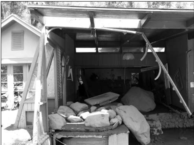
Photo 10. Home destroyed along Oak Creek. Photo by Dave Wagner.
