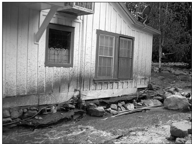
Photo 15. This cabin on Oak Creek was damaged by mud, but cleaned and made habitable. Photo by Jim Stroh.
