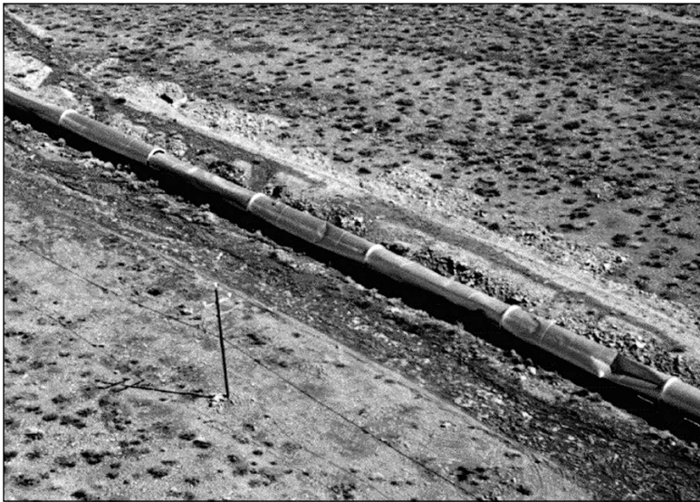
Figure 2-2. Collapsed aqueduct pipe, 1980s. [J. Westbrook photo]
