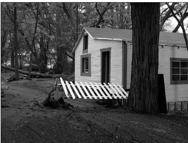
Photo 16. This house was damaged by inundation and the foundation undermined after partial realignment of Oak Creek. Photo by Jim Stroh.
