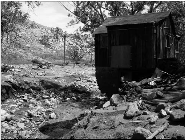
Photo 12. Remnant of the old Parker Ranch buildings along south Oak Creek. Note deep incision of new channel. This partial structure is all that remains of ranch buildings present prior to the mud flow. See also Photo 2. Photo by Jim Stroh.
