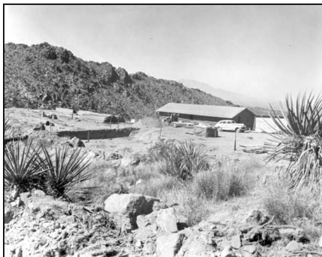
Vulcan Mine mess hall and foundation excavation for bunkhouses, August 1942. Photograph from the Bud Davenport collection, Mojave National Preserve.
