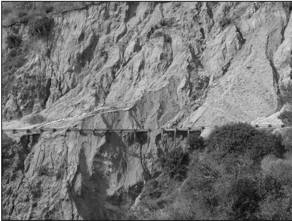
Figure 3. The Arcadia Slide looking west.
