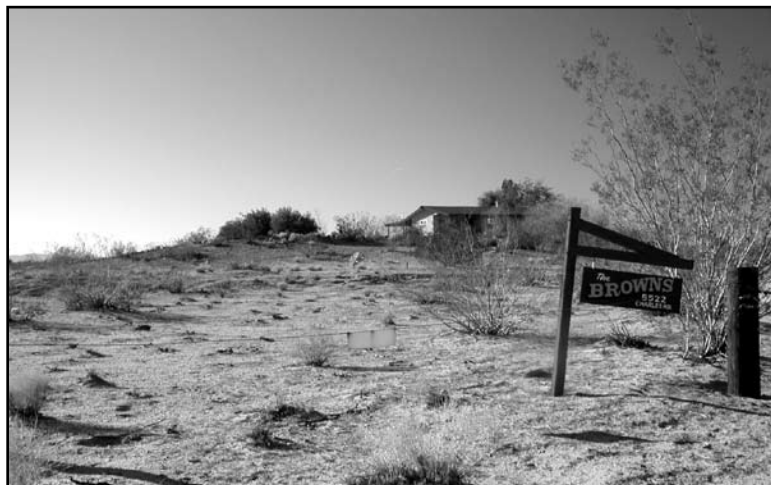
PHOTO 2-13, MP 137.9. View northwest of the Brown residence on Charles Road. A scarp up to three feet high produced a split-level front yard. The house sits on old graels that may indicate Pleistocene(?) uplift.
